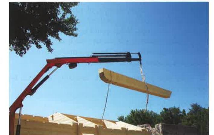
Figure 14.1 Network analysis can help building firms estimate when they will need materials and equipment
