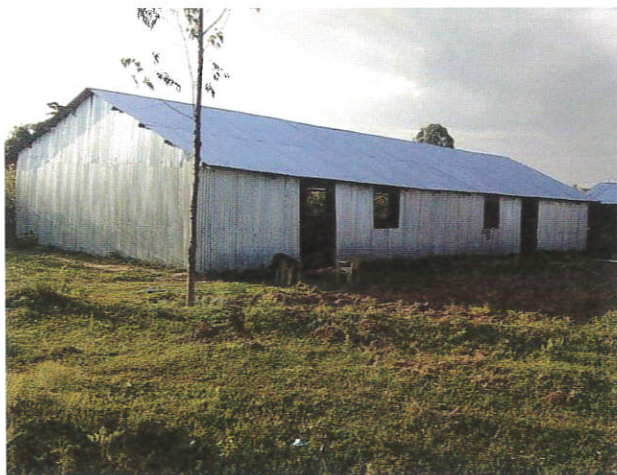
▲ A new church being built at Bungoma, in a rural part of Kenya, near the border with Uganda
